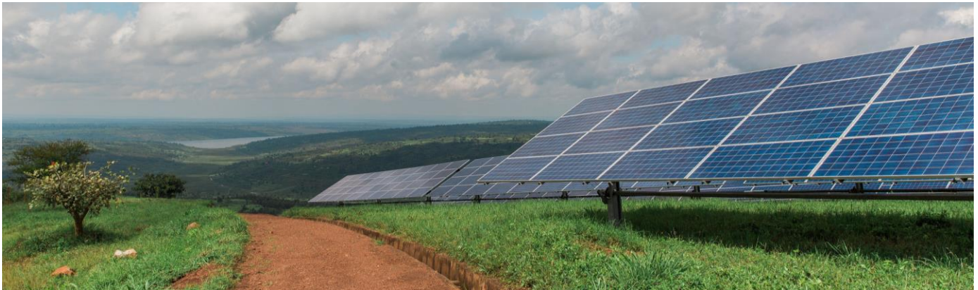
Solar installations like the Power Africa-supported Gigawatt Global Solar Field in Rwanda, the first utility-scale solar facility in East Africa, offer a path to clean energy solutions across Africa. (Photo: Rachel Couch for Power Africa)
