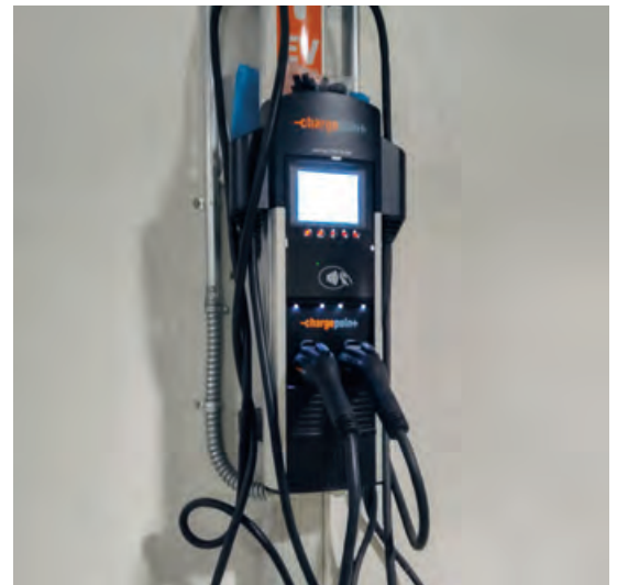
USAID's dual-port EV charging station in the garage of its USAID Annex Headquarters facility in Washington, D.C. PHOTO: USAID
