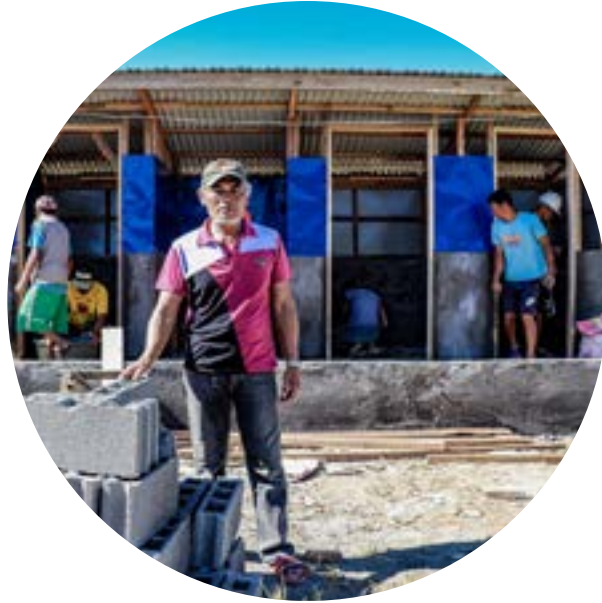
With support from BHA partner CRS, workers build latrines and bathing facilities in the Philippines' Lanao del Sur Province to support families displaced by the 2017 conflict in Marawi city. Photo courtesy of CRS
