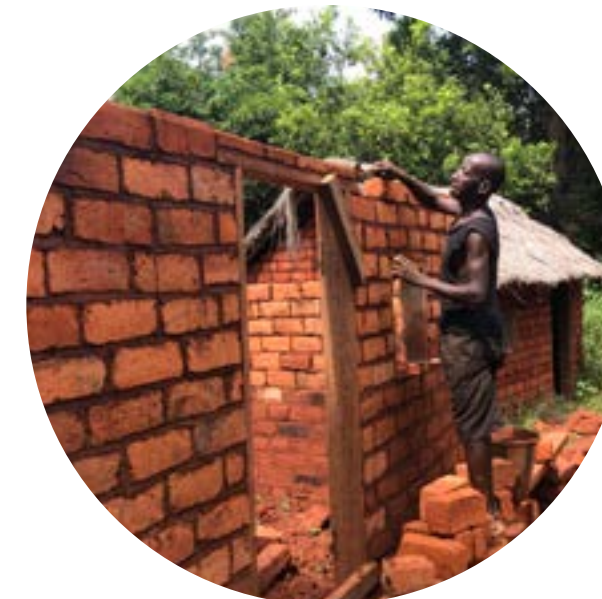
A man works on his transitional shelter in Zemio, CAR, utilizing materials provided by a BHA-funded partner. Photo by Dimitri Obolensky/USAID
