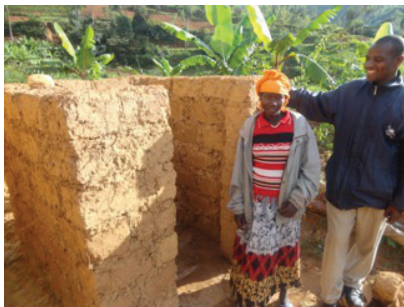
A pastor explaining the construction of a latrine with one of the members of his community. He explains that “building a latrine is not an easy task.”
