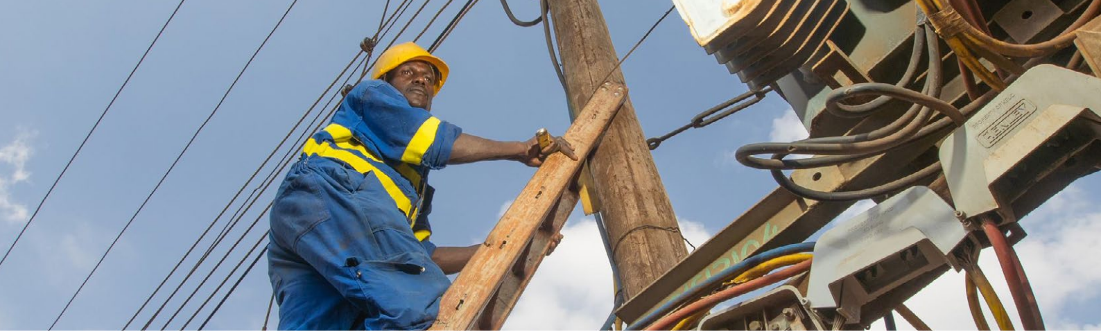
A technician inspecting a grid connection in Kasarani area, Kenya. (Photo: Mwangi Kirubi for Power Africa)
