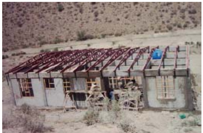
When complete, this USAID-funded clinic at Shewak village in Paktia province is 50% constructed, and will provide services similar to that of the clinic in Badakshan province.
